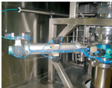
Sampler system for automatic collection of chemical powder.
