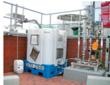
After: Automatic system for adding acid.
